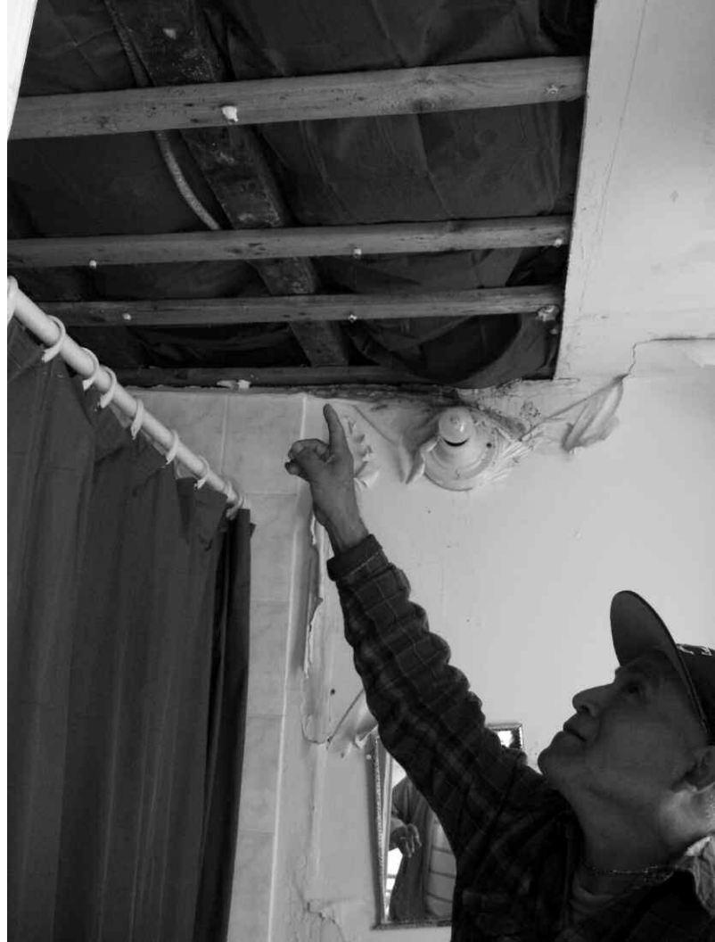
Fabian Rivera showing organizers a dangerous ceiling hole in the bathroom of his Bed-Stuy apartment building, one of 192 housing code violations in the building. Photo: Make the Road New York
